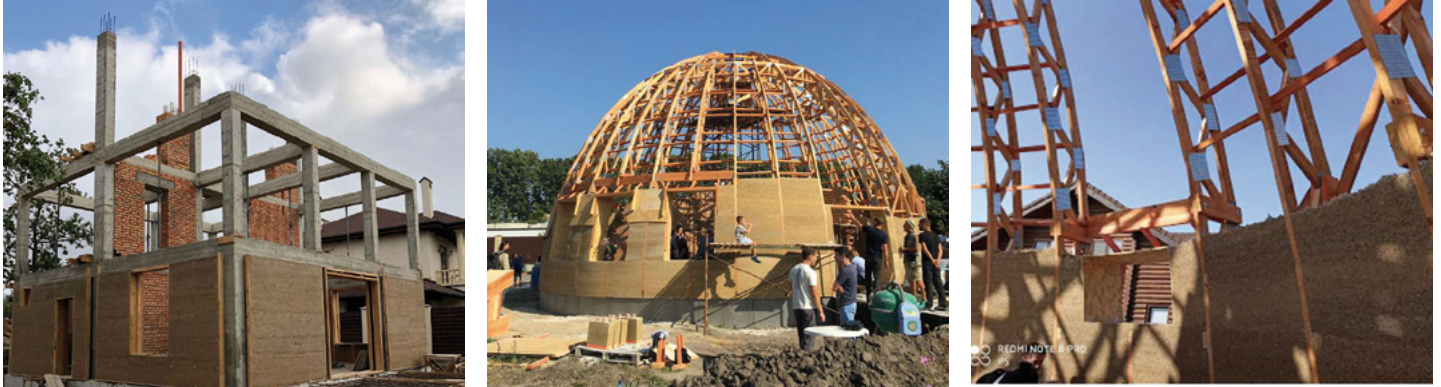
Fig. 13–15: Various building forms made of hempcrete, from cubic to vaulted structures in construction © Hempire
