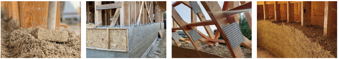
Fig. 9–12: Production and installation of hemp building materials: Mixing, compacting and filling hemp lime in timber frame constructions © Hempire
