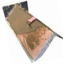
Fig. 21: Clay-soaked jute sacks on formwork and finished element © Leon Zimmermann / Institute for Architecture-Related Art, TU Braunschweig
